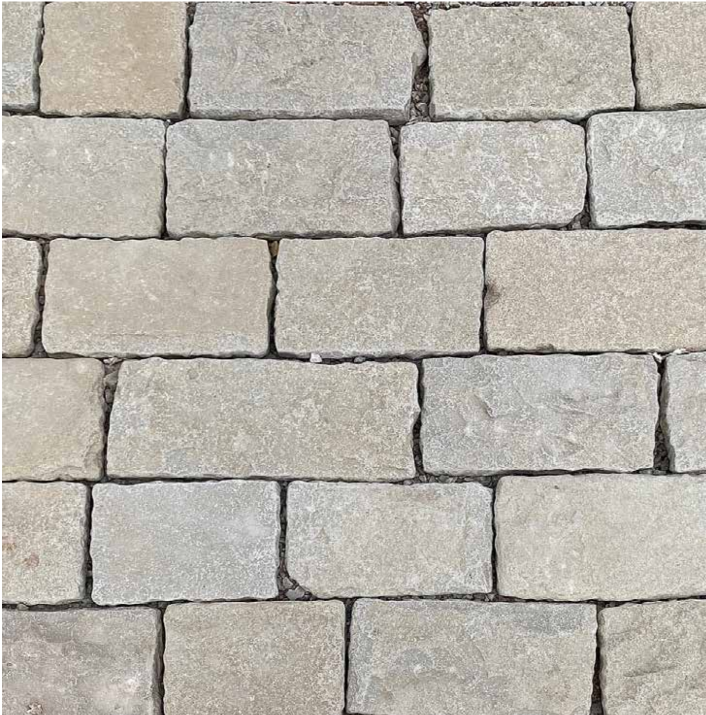
T.A.B. - Driveway - Old century driveway with uneven surface
